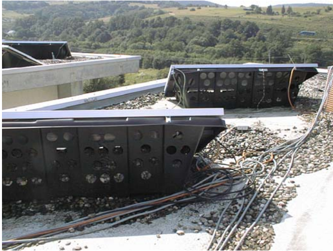
Fig. 7: test system is mounted on ventilated troughs
